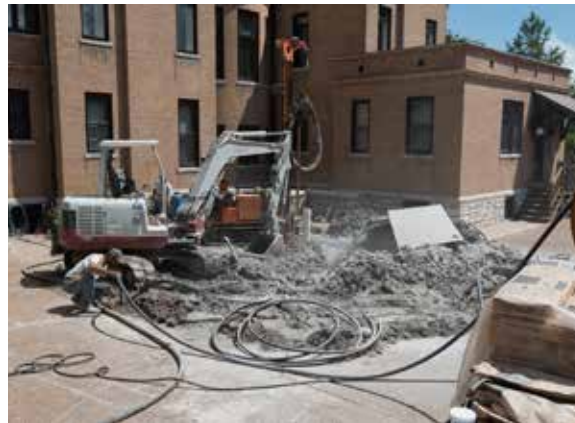
Left: Installation of the geothermal loops took place in the courtyard at the back of the mansion.
